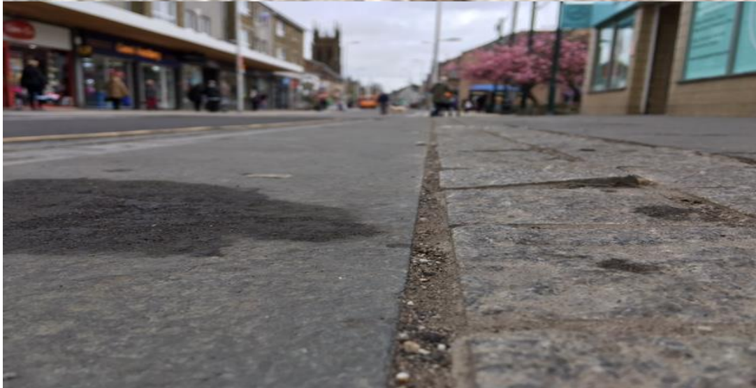
Photographs 8 to 10 Rough cobbles used along the entire length of the Cowgate scheme. Trip hazard to pedestrians and problems for wheelchair users.
